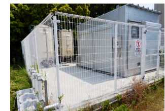
Groundwater membrane filtration equipment (Okazaki Plant)
