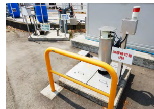
Surface oil detector (Okazaki Plant)
