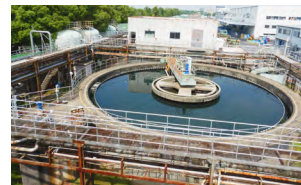
General effluent treatment facilities (Okazaki Plant)
