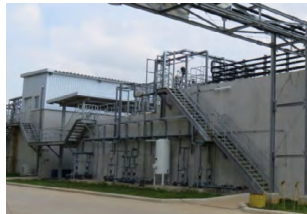
Industrial water and wastewater treatment plant (Indonesia)
