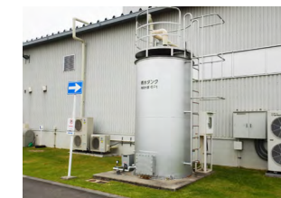
Rainwater storage tanks (Okazaki Plant)
